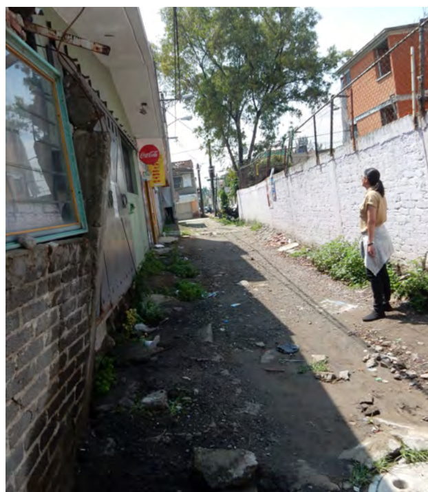
Our researchers examine the conditions of inhabited buildings one year after the 19-S earthquake in Mexico City. Photo: IDMC/Vicente Anzellini, September 2018
