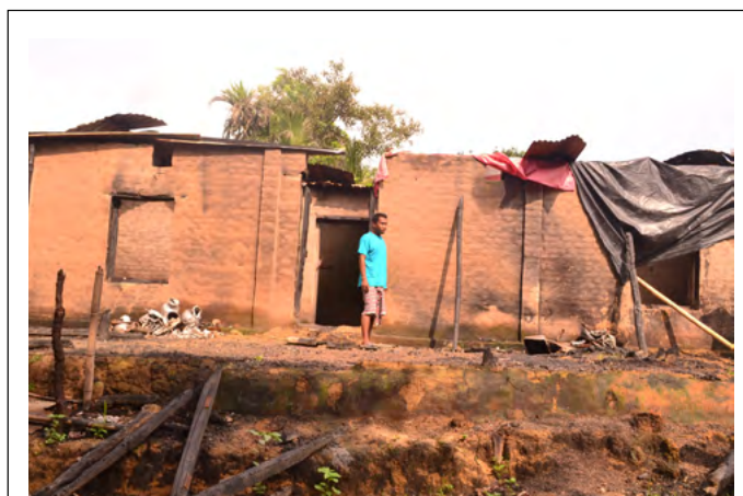
House set on fire during inter-communal violence in August 2013 near Taindong Bazar of Matiranga Upazila in Khagrachari District. Its Pahari inhabitants were among those forced to flee. Photo: (c) Mita Nahar, August 2013
