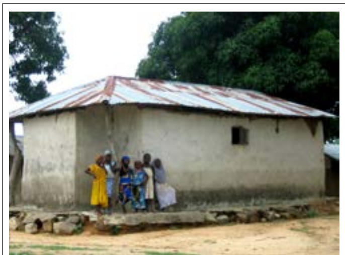
Girls standing in front of a water-damaged house in Gurmana, Niger state, which has flooded every year for decades. During the 2012 floods, the whole village had to temporarily relocate to the primary school. Photo: IDMC/Noémie Pierre, May 2013
