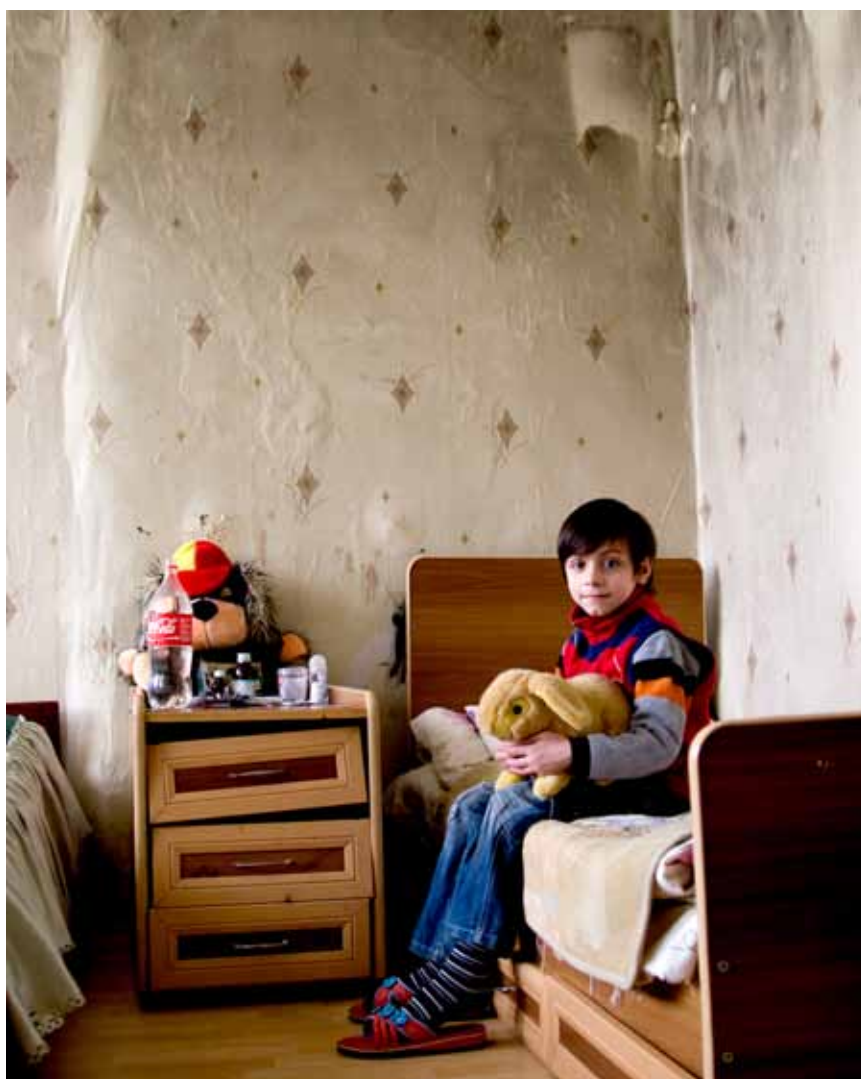
A seven-year-old child, whose family was displaced from Gagri, Abkhazia, has lived in this shelter in Greater Tbilisi, Georgia, since birth. The building is in a poor state of disrepair. (IDMC/Daron D'Souza, 2011)
