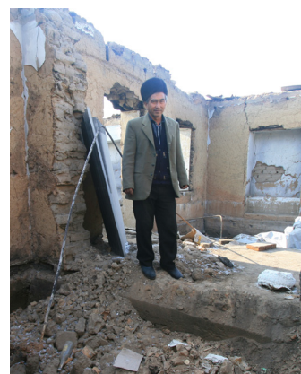
The extent of the damage done to this returnee's house means he must rebuild his home from scratch, Kyrgyzstan. (IDMC, January 2011)
