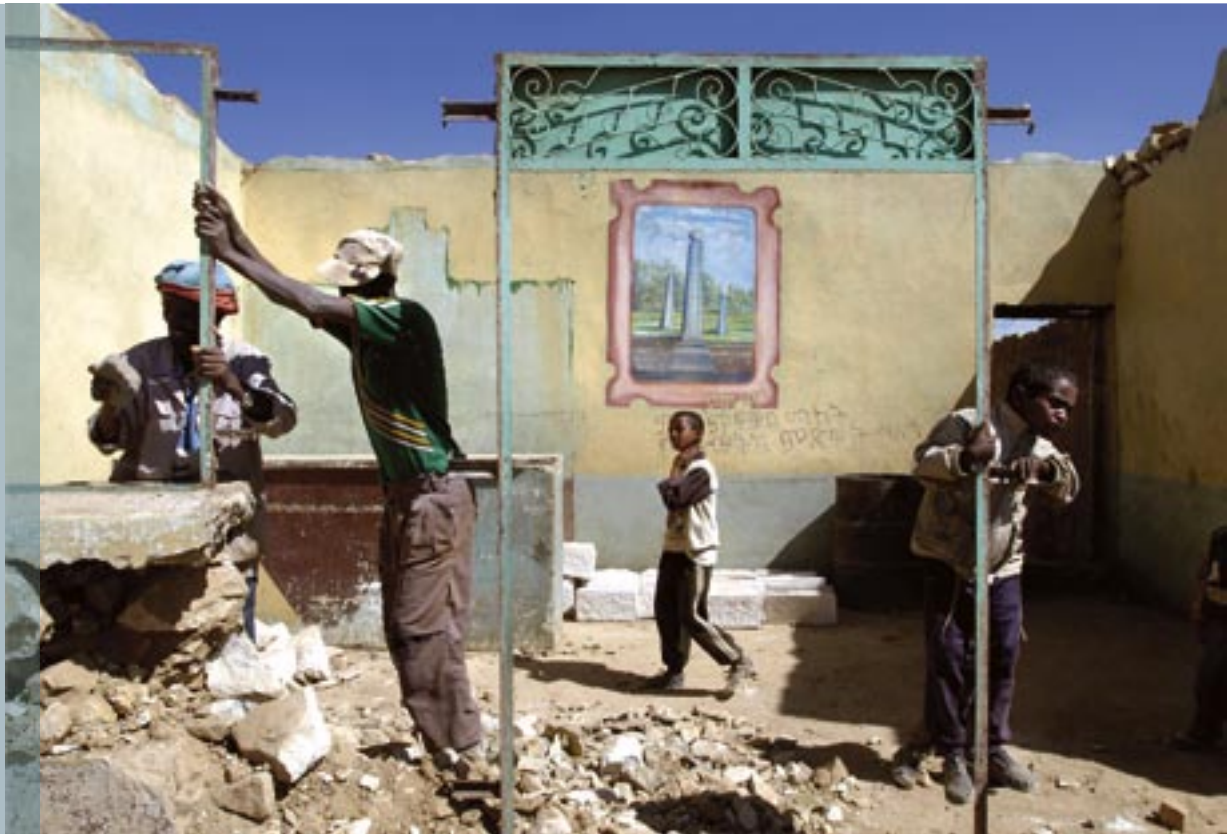
Ethiopian returnees rebuild their house, destroyed during the Ethiopia-Eritrea border war. (Photo: Sven Torfinn, Panos)
